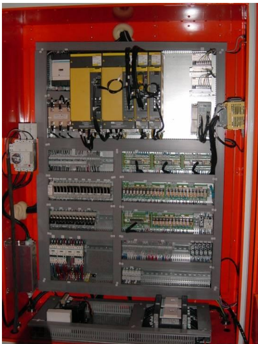
Fig. 47 Electrical cabinet w/Fanuc control
