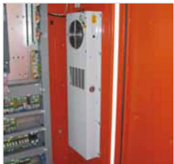
Built-In Heat Exchanger
