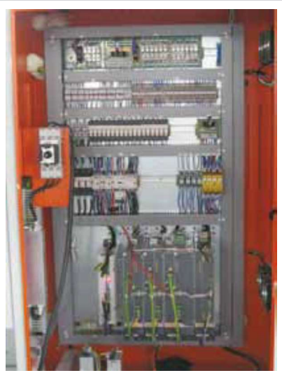
CE-Marked Electric Cabinet
